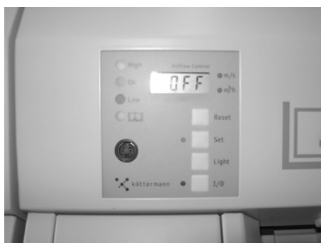
Fig. 7.: Display of the hoods in room A 317
