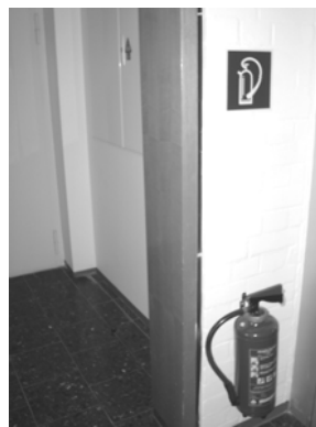
Fig. 3: Powder fire extinguisher in front of fuse boxes of electric power supply
