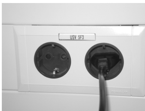
Fig. 6.: Red power outlets of the UPS
