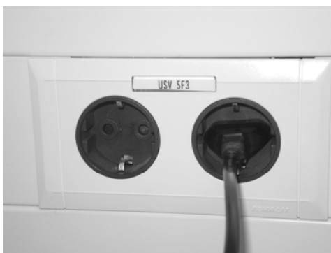
Fig. 6: Red power outlets of the UPS
