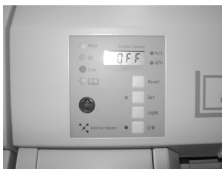
Fig. 7.: Display of the hoods in room A 317
