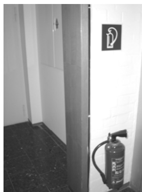
Fig. 3: Powder fire extinguisher in front of fuse boxes of electric power supply
